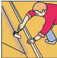
Apply primer with a brush or roller and allow to dry. (See above for details)
